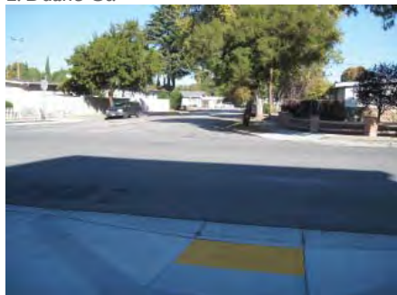
Some intersections lack curb ramps. Curbs are often located in the middle of the corner. Some curbs lack associated crosswalk.
