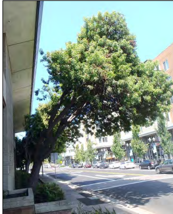
Photo 1: Looking west at Brazilian pepper #286. The tree was typical of the Brazilian peppers growing along the north side of the Macy's building. It leaned and had a one-sided crown to the north as a result of pruning/topping for building clearance and phototropism.
