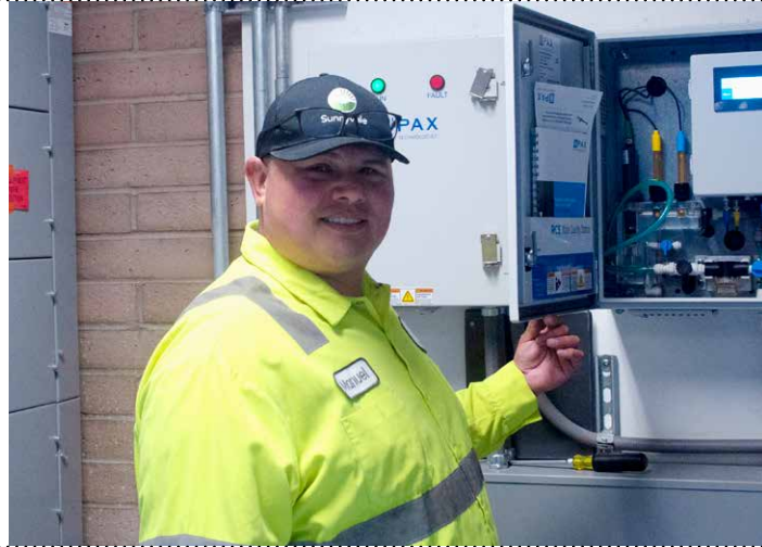
Senior Water Distribution Worker Manuel Hernandez checks water pressure and chlorine levels at the City's pump stations.
