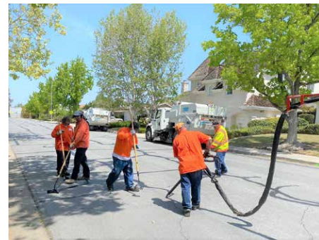
Our Street Operations team – including Eric Cervantes, Adam Leros, Ray Hernandez, Justin Driscoll and Rick Diaz – perform pavement maintenance on over 260 miles of Sunnyvale streets.
