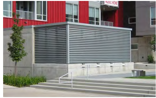
Screen mechanical equipment visible to the public and integrate into the building architecture.
